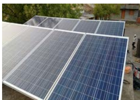
Solar Energy Panel at Bolegaon Village
